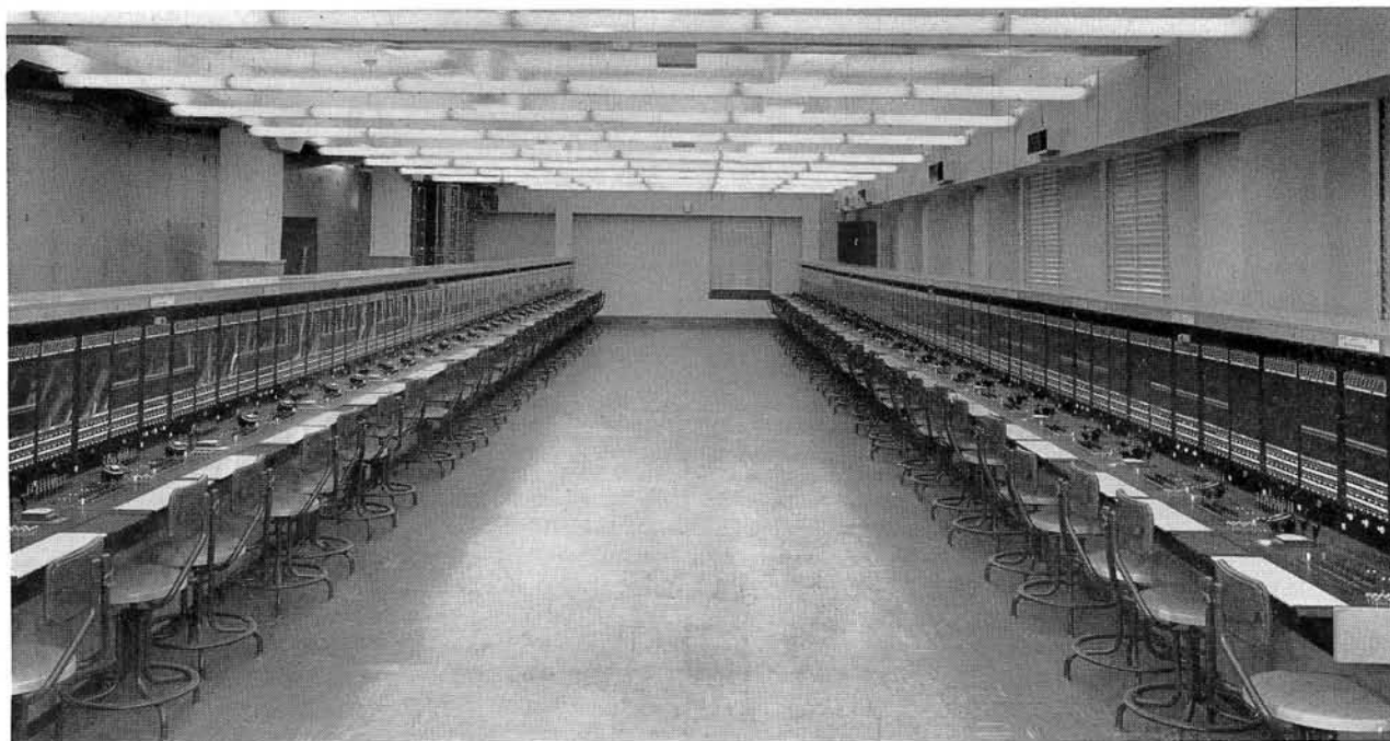
80 Positions of Stromberg-Carlson No. 3 Toll Switchboard in a large toll center.
